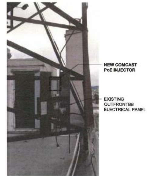
VIEW OF EXISTING OUTFRONTBB ELECTRICAL PANEL
